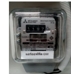
The electrical meter measures the complete electrical consumption of the A/C system (Indoor unit + outdoor unit).
