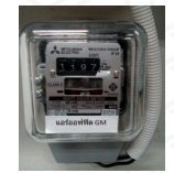
The electrical meter measures the complete electrical consumption of the A/C system (Indoor unit + outdoor unit).
